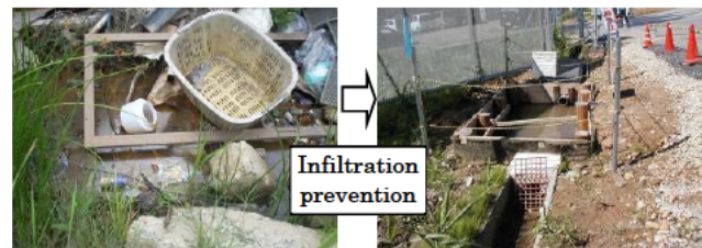
Photo 6. Water-treatment installation and pond for infiltration and environmental risk
